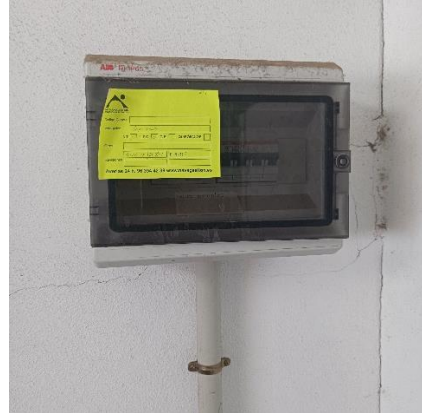
P.O. SECTOR 4 SALA SIST.CONTRAINCENDIOS
